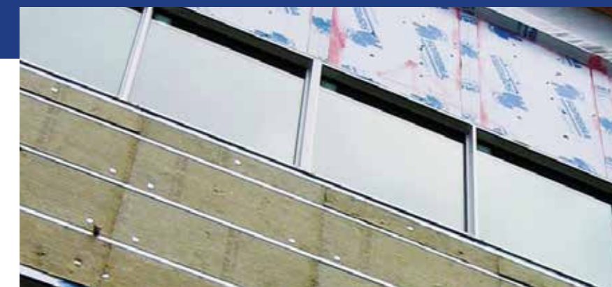
Exterior insulation installed in-between steel z girt cladding support attachment resulting in exterior insulation that is not continuous and does not meet energy codes (Source: Roxul, Inc.)
